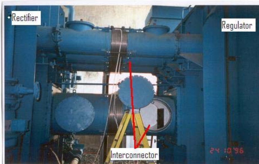
Figure 11-Interconnection system for the Rectifier and Regulator Transformers.
