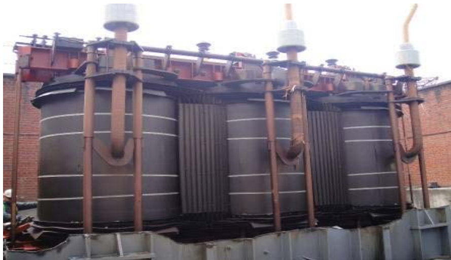
Figure 3-Three winding assemblies on core, HV side view
